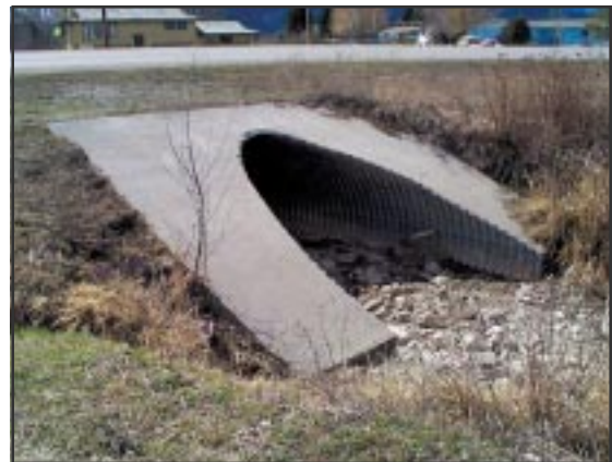
This arch pipe is sized to carry the predicted 25-year flow, but causes backwater at the 100-year flow.
