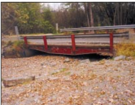
A low stringer in an aggrading channel does not leave much room for water. Note that the beam hangs low in the center and restricts peak flow capacity and debris passage.
