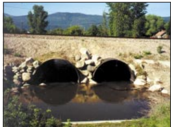
A half-hearted effort at armoring the inlets, but note that the pipes are set below grade, which is good for fish passage.
