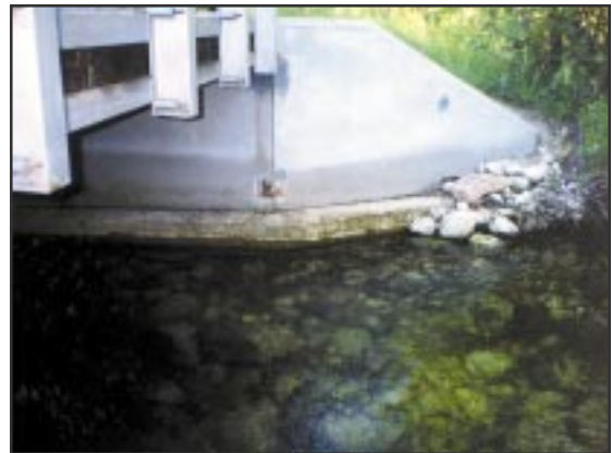
Concrete can make good abutments, provided the footing is placed below scour depth. This footing should be 2 feet lower.
