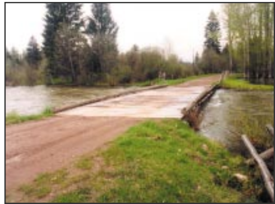
Stream crossings on shallow channels with broad floodplains must rise to meet the bridge, or the bridge will end up being too low, like this one.
