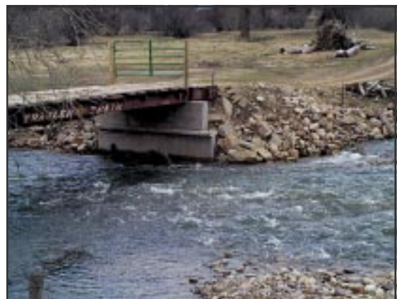
Stacked median barriers often make poor abutments. The absence of wingwalls, footings, and a 1:1 fill slope mean this bridge is likely to require additional maintenance.
