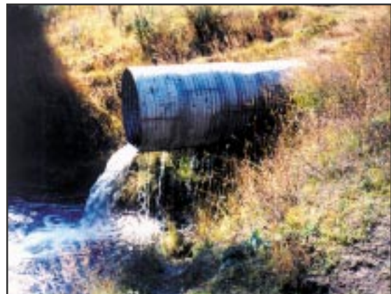
The shotgun (or perched outlet) culvert impedes fish passage, and can result from placing the culvert too high, or installing the culvert in a channel that has a tendency to downcut without grade control downstream of the outlet.
