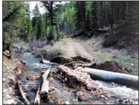
Undersizing pipes to save money is a poor strategy.
