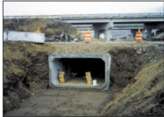
Concrete box pipes frequently have poor fish passage characteristics because of the smooth, flat bottom.
