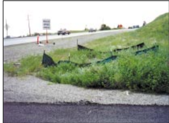
Silt fence helps prevent sediment delivery on newly constructed roads, but does not substitute for proper drainage features.
