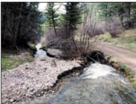
Aggradation from a failed culvert crossing has decreased channel capacity and increased flood risk to the road that has encroached on the floodplain.
