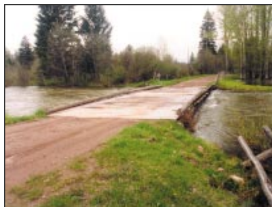
This bridge stringer is set at bankfull height. Projects should avoid this situation, which traps debris.
